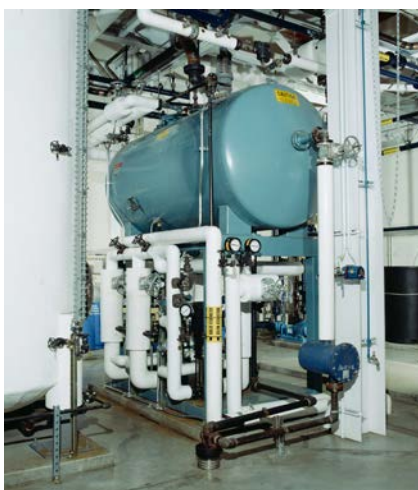
Figure 4 Deaerator (DA) tank in boiler room
