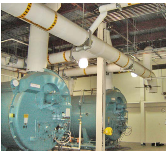
Figure 2 – Boiler header in a healthcare facility
